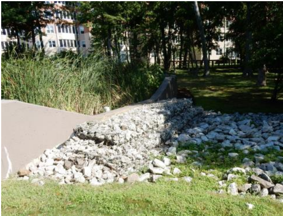
Existing Pond at BayWoods of Annapolis Overflow Weir and Outfall Protection (facing northwest)
